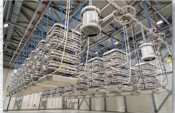
HVDC Light® NordLink (1,400 MW / ±525 kV)
